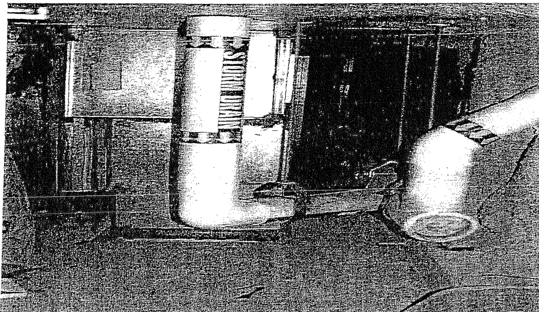
Photo 15: Cable Access Room (CA1).
