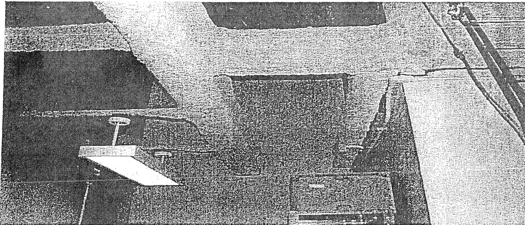
Photo 49: Yellowed Fireproofing, Intermediate Level Beam, 7TS5.
