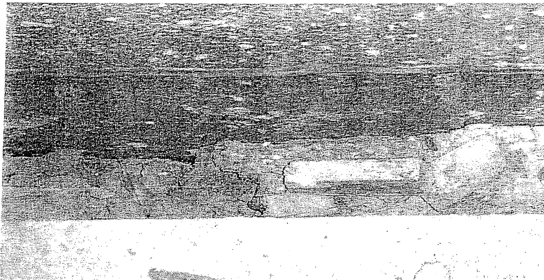
Photo 31: Debris found in 11 th Floor Outer Ring.
